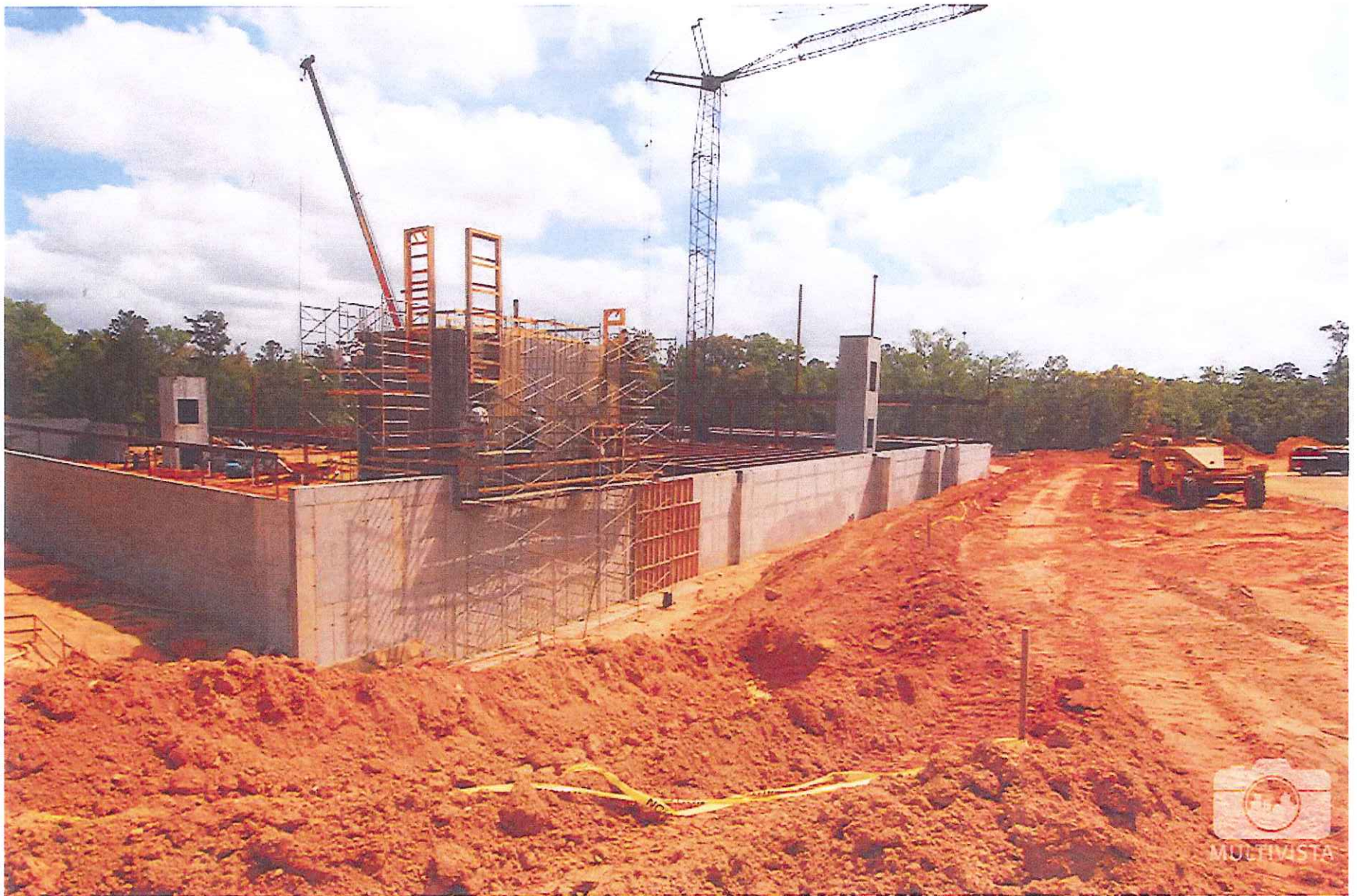
Tallahassee Community College - TCC Ghazvini Center for Healthcare Education - 1528 Surgeons Dr - Exterior Progression - - April 7 2010 - Photo Number 3
